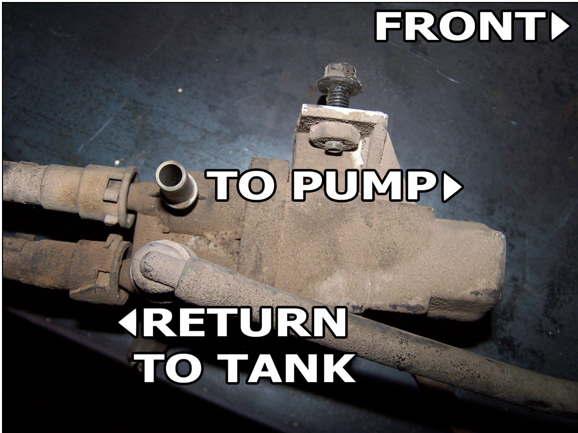
Figure 5 – Fuel Tank Selector Valve – RETURN HOSE Identification
